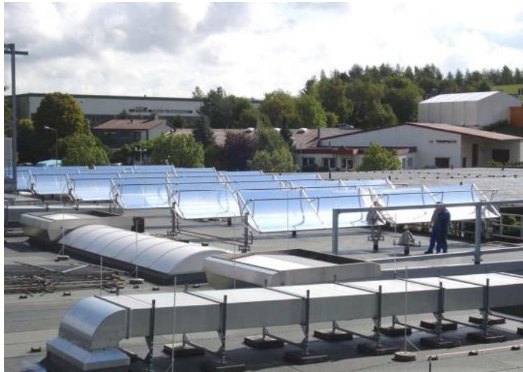
Fig. 20. Alanod PTC facility (Lauterbach, n.d.).
